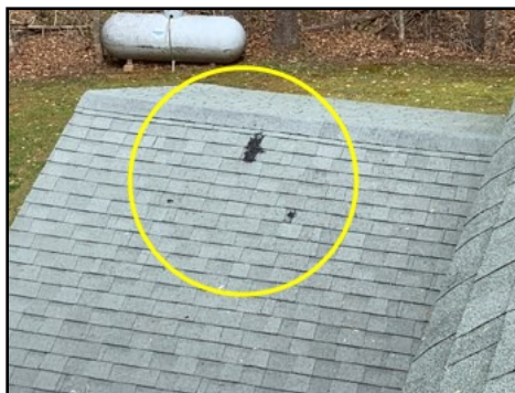
Tar Repair Observed
