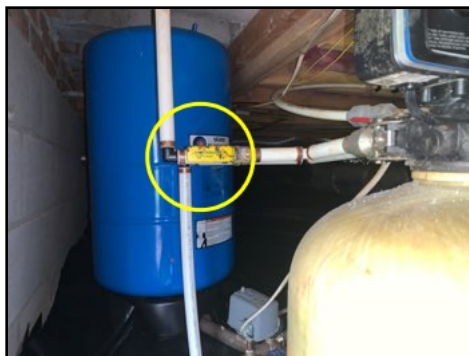
This is the main water valve in the crawlspace.
