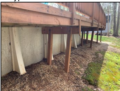
Leaning Deck Posts
