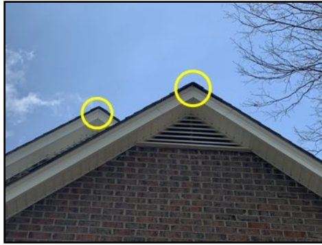
Torn Shingles Observed Here
