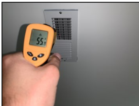
Supply Air Temperature Second Floor (55.9)
