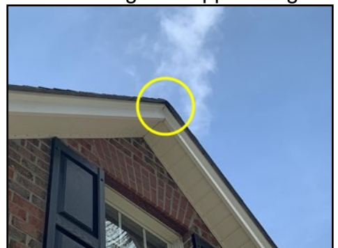
Torn Shingle Observed Here
