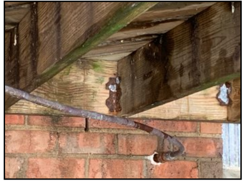
Rusted Joist Hanger (Representative Photo)
