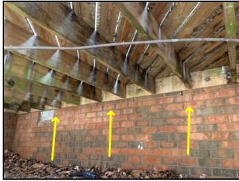
No Ledger Flashing Observed
