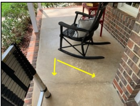
Typical Crack at Front Porch
