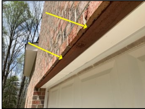
Rusted Lintel (Representative Photo)
