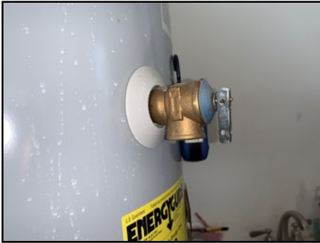
Missing Discharge Pipe (Water Heater TPRV)
