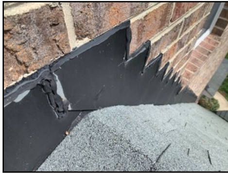
Worn Sealant at Counter Flashing (Representative Photo)
