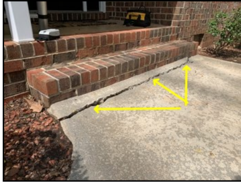
Some Settlement Observed (Front Walkway)
