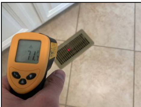
Emergency Heat not Operating Properly
