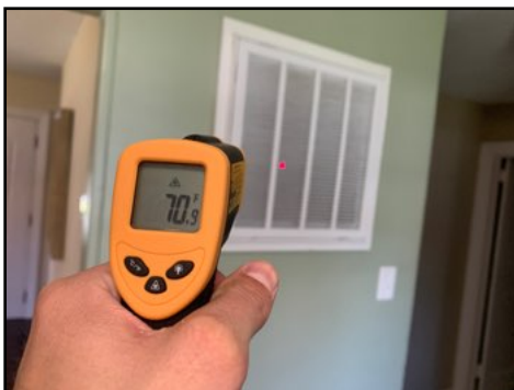
Return Air Temperature (70.9)
