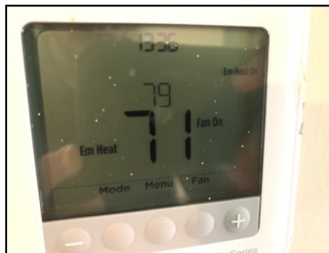
Thermostat set to Emergency Heat
