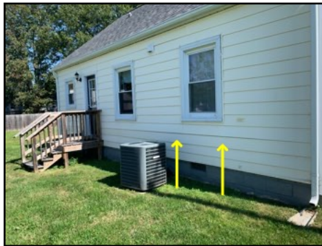
Loose Siding Observed Here
