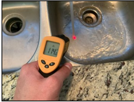
Hot Water Temperature (114.6)
