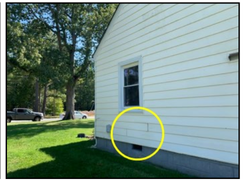
Caulking/Inadequate Sidelap Observed Here
