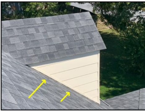
Example of Vinyl in Contact with Roof
