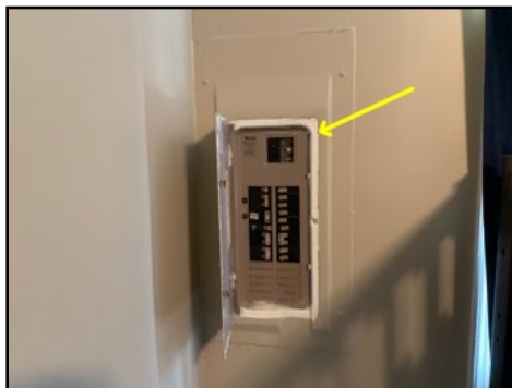
Main Disconnect Location: Rear Left Bedroom
