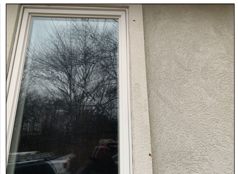
Damage Observed (Forward of Garage Doors)
