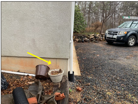
Typical Crack Observed
