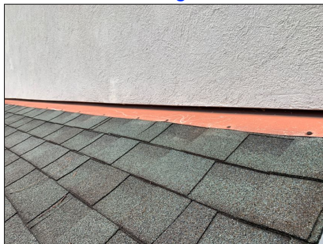
Exposed Nails Observed
