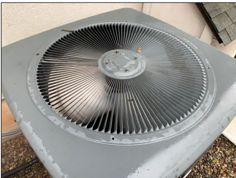
First Floor & Basement AC Operating in Cooling Mode
