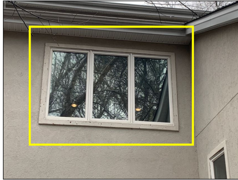
Damage to Siding Observed at This Window
