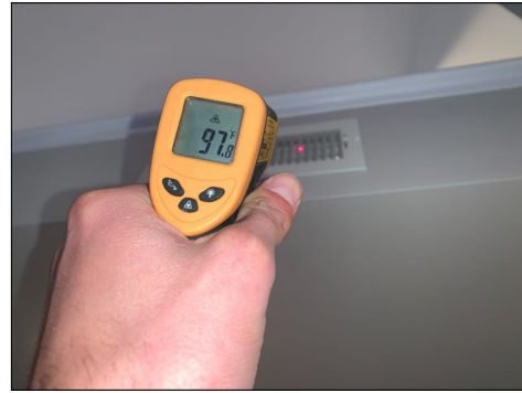
Second Floor Heating System Functional (97.8)
