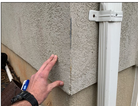
Crack at Corner (Rear of Garage)
