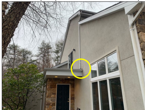
Downspout Terminating Above Roof
