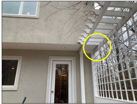
Rot in Soffit Observed Here
