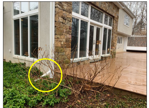
Downspout Terminating too Close to Foundation
