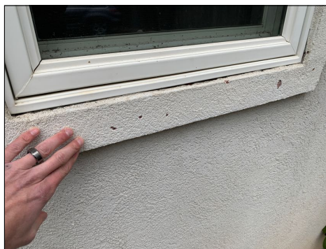
Damage Observed (Forward of Garage Doors)
