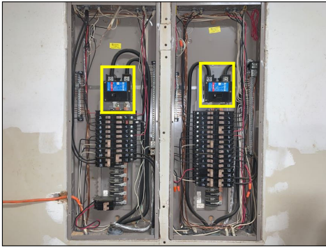
Main Disconnect Location: Garage
