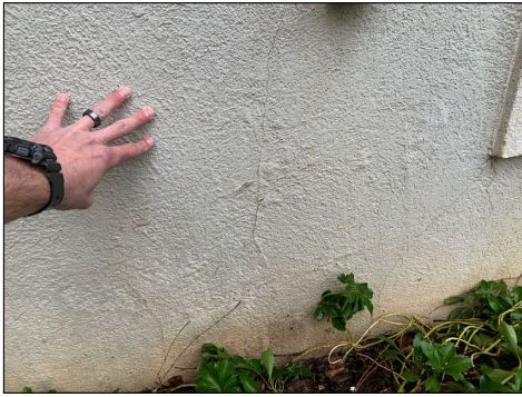
Cracks/Spalling Observed (Near Front Door)
