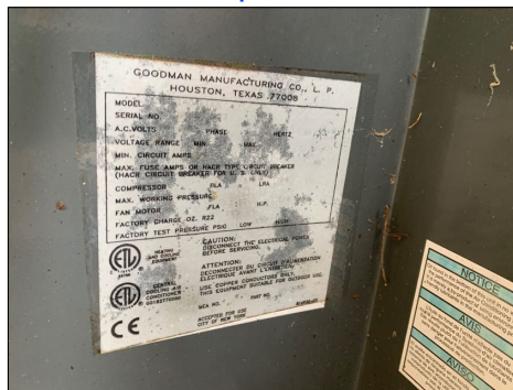
Data Tag (First Floor & Basement)
