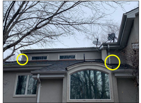
Downspouts Terminating Above Roof
