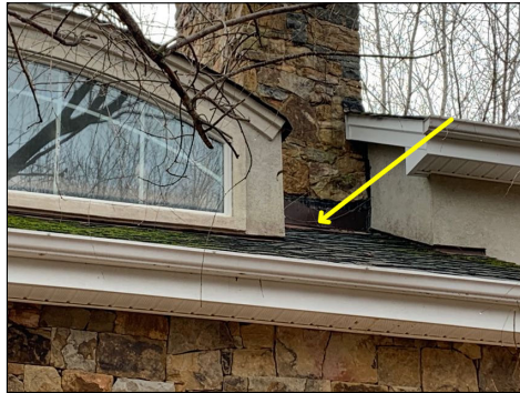
Evidence of Leak Observed Here
