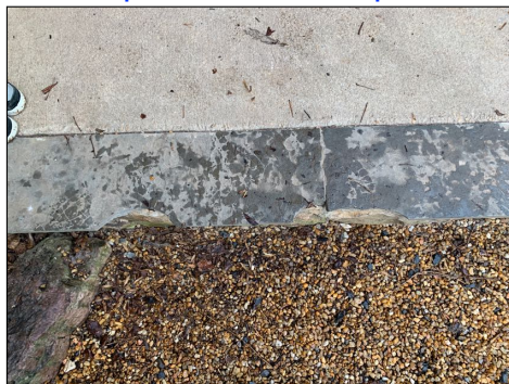
Damage Observed at Front Steps
