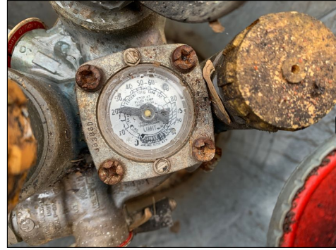
Remaining Propane in Exterior Tank
