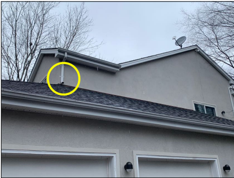
Downspout Terminating Above Roof
