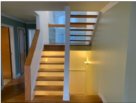
Open Risers Observed
