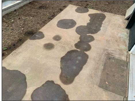
Leaks Observed in Solarium
