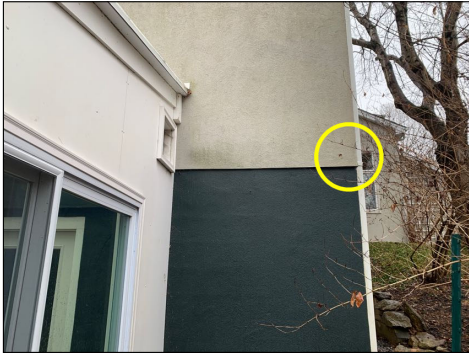
Damage to Siding Observed Here
