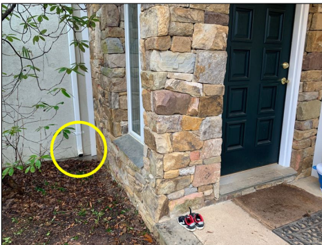
Downspout Terminating too Close to Foundation
