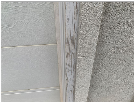
Peeling Paint Observed (Representative Photo)
