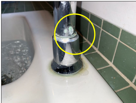
Leak at Kitchen Sink Faucet
