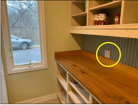
This Outlet in the Utility Room had a Reversed Polarity Reading
