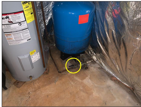
This is the main water valve in the basement.
