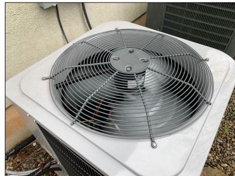
Second Floor Heat Pump Operating in Cooling Mode
