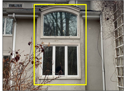
Damage to Siding Observed Around These Windows (Rear of Home)
