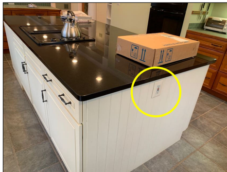
This GFCI Device did not Trip when Tested
