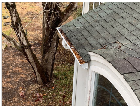
Gutters Full of Debris (Representative Photo)
