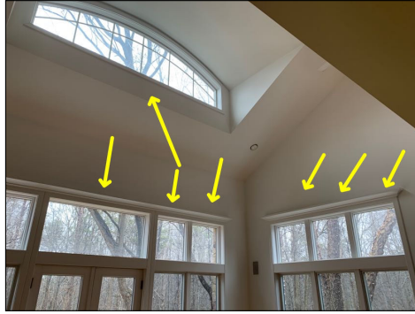
These Windows in the Living Room had Condensation Between the Panes
